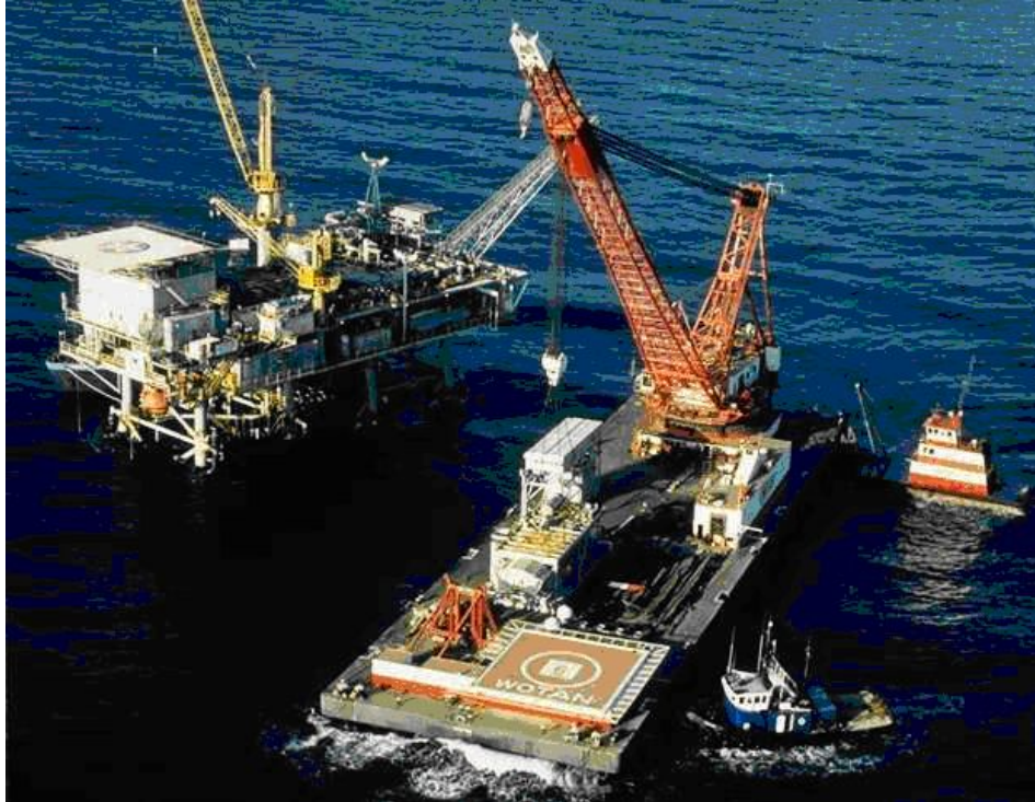
Figure 18 - Manson Construction 600 ton Derrick Barge WOTAN operating offshore In heavy currents these barges use a mooring spread that allows them to keep on station and accurately reposition themselves continuously using hydraulic winches controlled by the operator.
